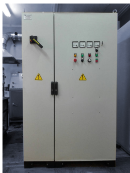
Thyristor and transistor converter of 5th generation with industrial internet function 第五代具有工业互联网功能的晶闸管-晶体管变流器
